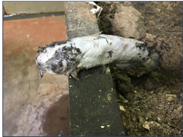
Figure 1 - Fish Caught on WWTP Bar Screen
